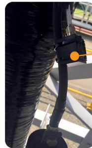
TM Sensor on Cable Termination
