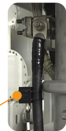
TM Sensor on GIS Cable Termination
